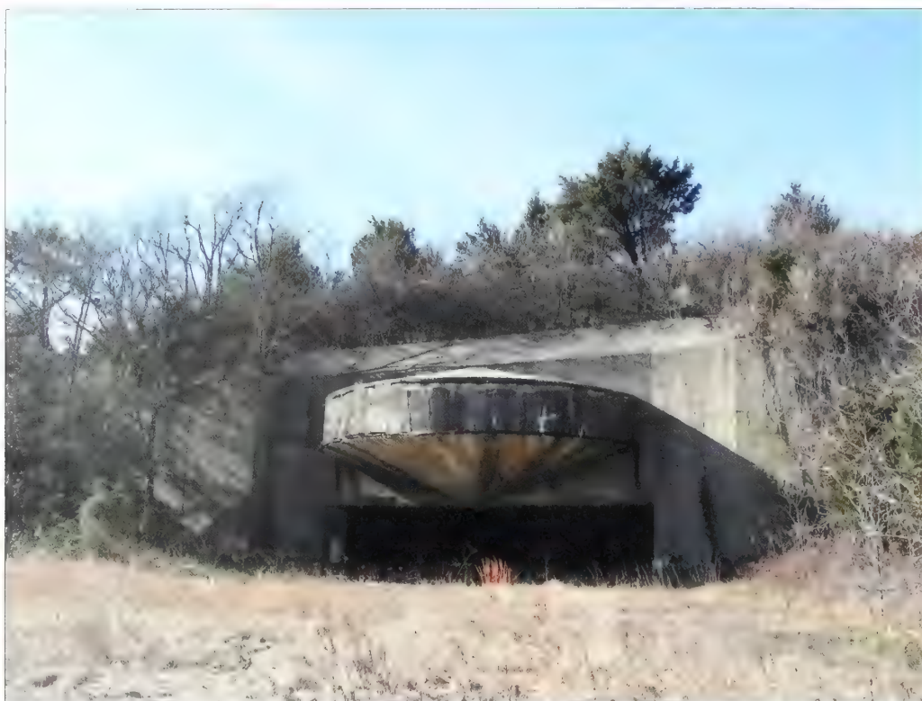
Figure 5.85. View looking southwest at north gun emplacement, Battery Kingman. Although visitors are warned of the hazards of accessing the summit of these batteries, existing chain-link fencing located above the concrete casemate canopies should be maintained for added safety at both Battery Kingman and Battery Mills (Olmsted Center, January 2009).
